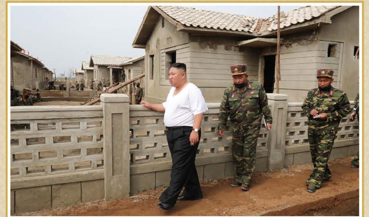
Kim Jong Un gives on-site guidance over construction in the flood-hit Taechong-ri area, Unpha County, North Hwanghae Province, in September Juche 109 (2020).
